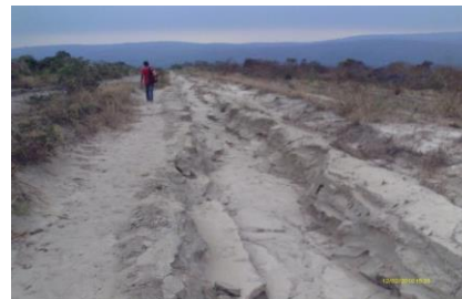
Photo 4 : Evolved gutters at the exit of Case Barnier
